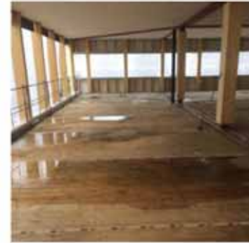
Fig. 5. On several occasions, water pooled on the floor structure. Precipitation ran down primarily from the above floor structures.
