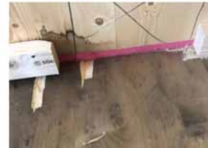
Fig. 8. Sample taken from the top side of the floor structure (CLT) under the sound and vibration pads and inner walls (CLT). The surfaces have been stained primarily by discoloured water.
